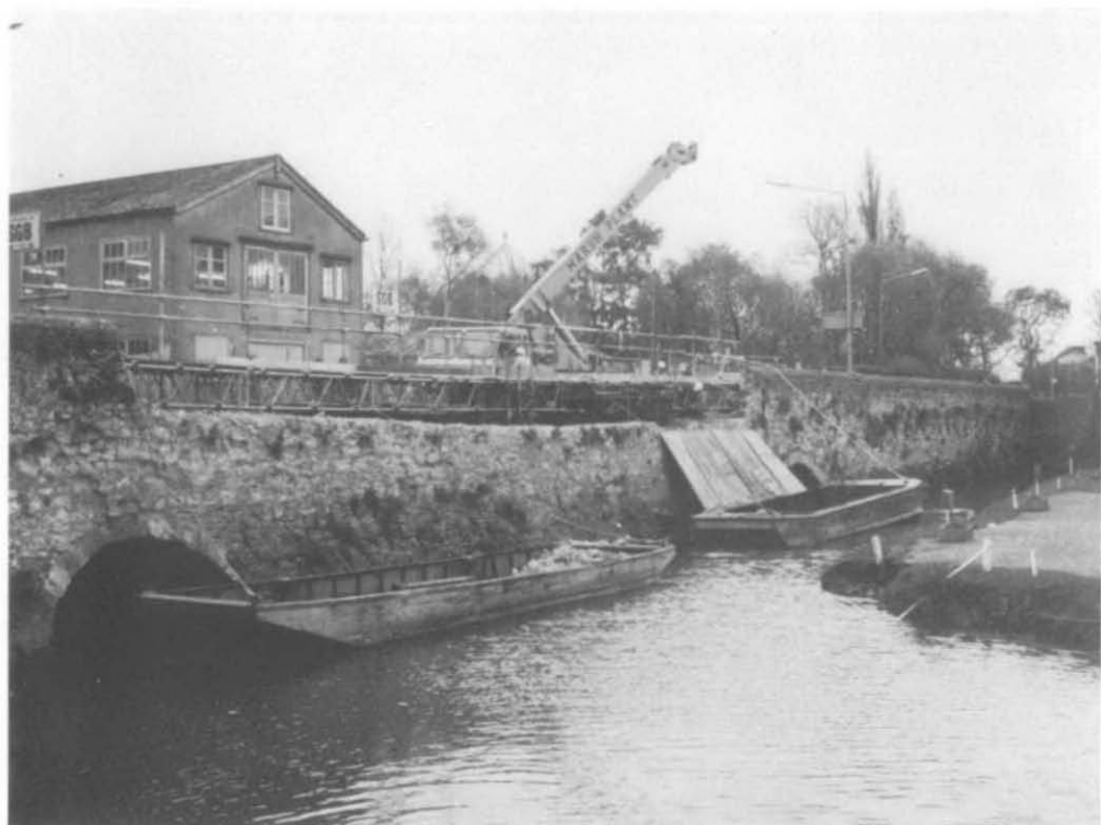
Plate 2. Causeway arches BNC 2-4 south of Folly Bridge viewed from north-west. The collapse of 1980 affected only the c. 18th-century stone skin of the second western widening, the Norman work being well protected in the core of the causeway.
