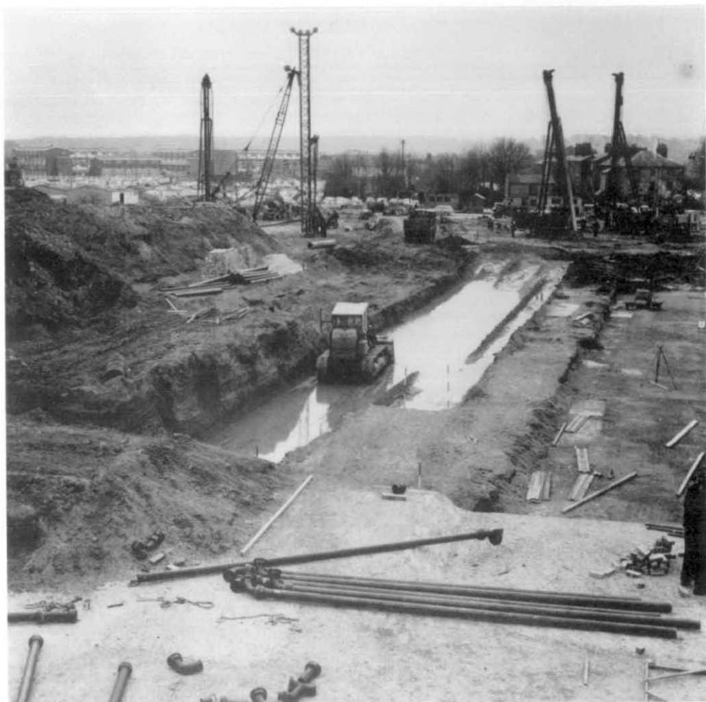
Plate 18. Westgate, Site W. Contractors' bulk excavation. The pits and wells can be seen cutting down through the natural gravel. View from the N. Photo by K.W. Sheridan.
